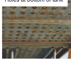
Holes at bottom of tank
